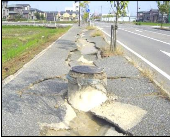
Cracks caused by an earthquake
